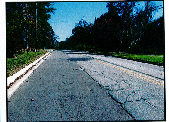
Road in need of resurfacing
