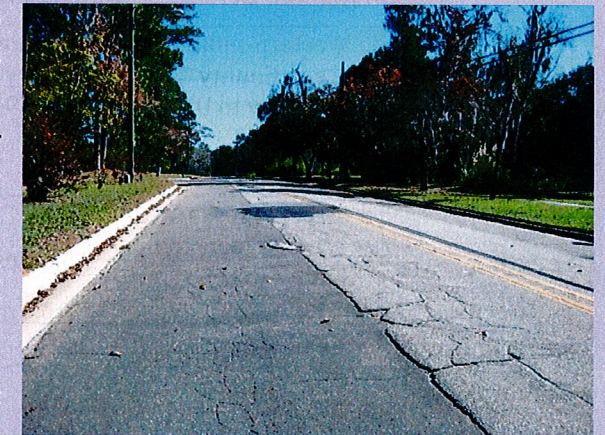
Pavement in disrepair on East Pearl Street Source: Jefferson County Studio
